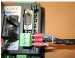
MAIN SCO 10 communication wire end
